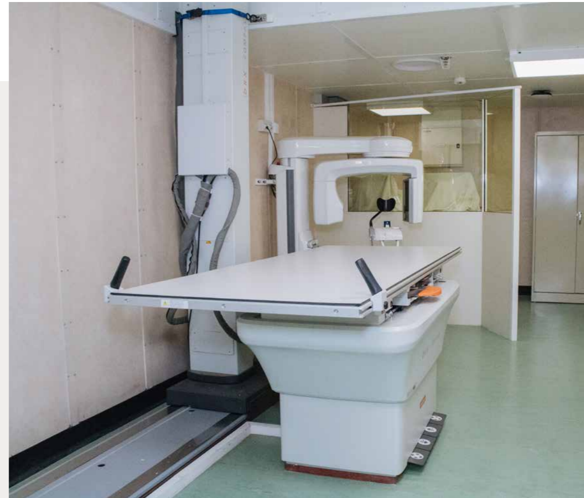
IMAGE: The installation of new X-ray and CT machines will enable advanced diagnostic photos, allowing medical crew on board to respond with enhanced speed and accuracy.
